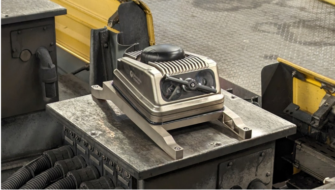
PANDAS-V® camera installed on a train roof
