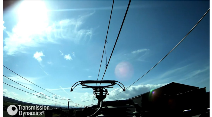
Broken Dropper Wire
